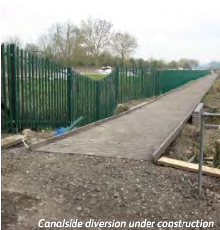
Diversion of a canalside public footpath with bridge culvert construction involving substantial fencing, drainage works and vegetation clearance
